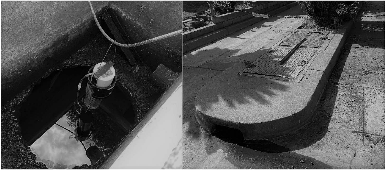
Figure 2. —The drain and two access lids to the double chambered BMP on Nada St. in the City of Downey (right). The drip system hanging in the inundated dry well (left).
