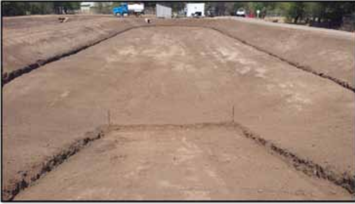
Figure 2: The pond bottom contours consist of a rounded trough down the center of the pond flanked by two flat walkways on either side, and a concrete launch ramp at the head.
