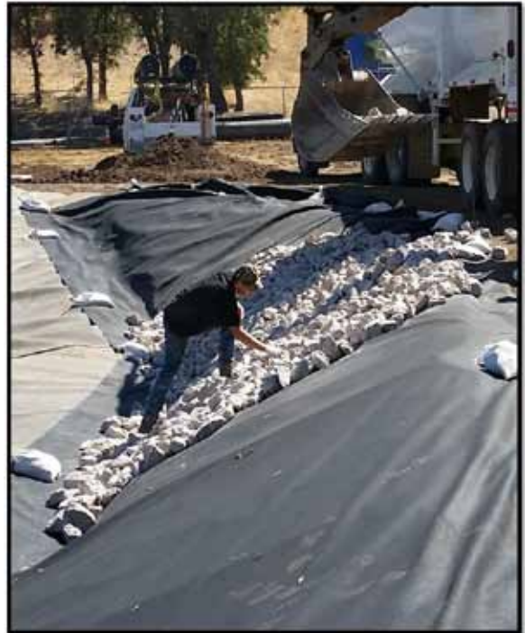
Figure 4: River rip rap rock installation. A felt liner was installed to protect the delicate pond liner and prevent rocks from slipping into the ponds.
