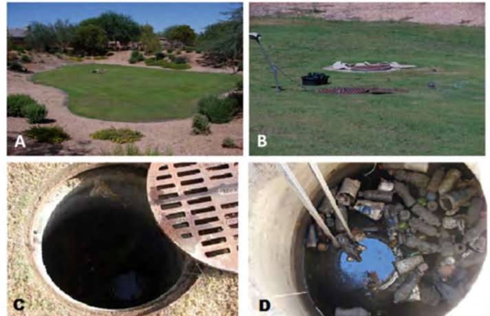
Figure 1. Maxwell® drywells were used to test the Mosquiron products. (A) Below grade grassed detention basin. (B) Multiple drywells within each detention basin. (C) Installed drywell. (D) Inside the drywell; the treatment area with stagnant water, organic debris and trash.
